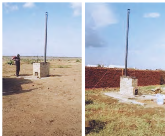
Figure 15 - Photos of double-chamber incinerator
